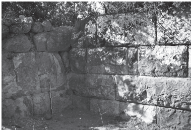
Fig. 20. Tower 10 . Detail showing the north wall of limestone ashlars meeting the curtain wall of soft, white andesite.
