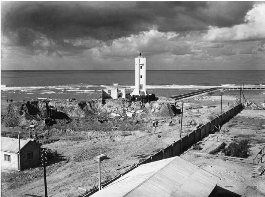
Fig. 43. Mechanical works cutting and damaging the mound of Tell Qudadi (1937), looking west (photograph: unknown; IEC, historical archive section).
