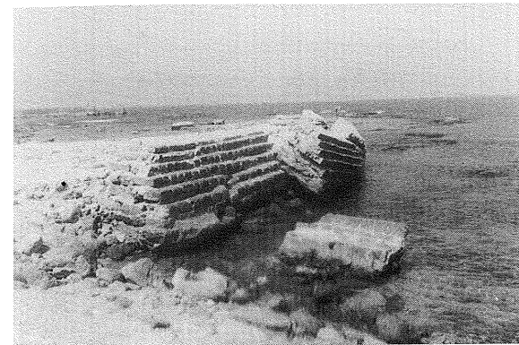
Fig. 45. A modern mole, built in 1961, in Caesarea, in an advanced stage of deterioration due to the undercutting and suction of the waves.
