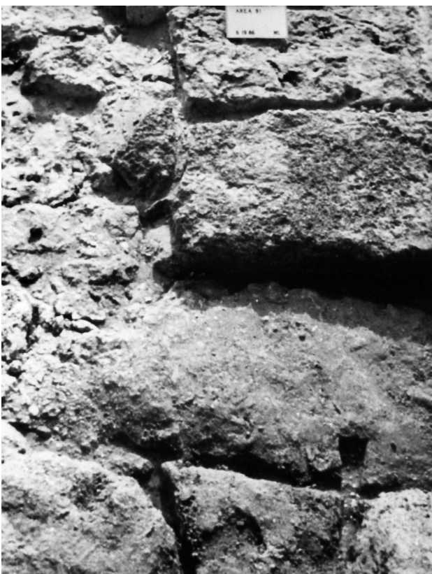
Figure 5.83. Dovetail grooves for metal clamping at the stem of the pier in Area L (Photograph: A. Raban)
