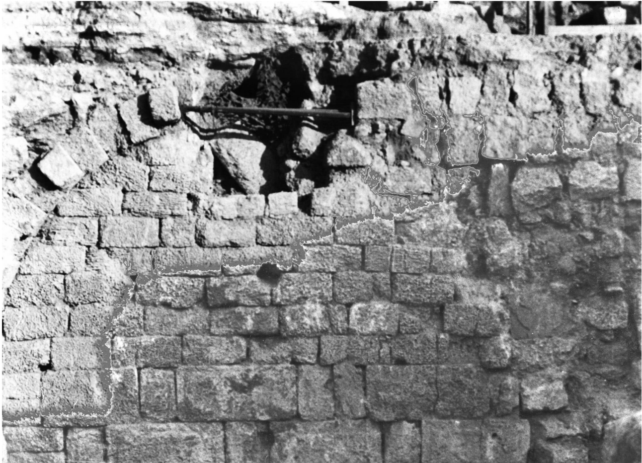
Figure 2.34. The backwall of IAA vault 3, looking towards the east. (Photograph: A. Raban)
