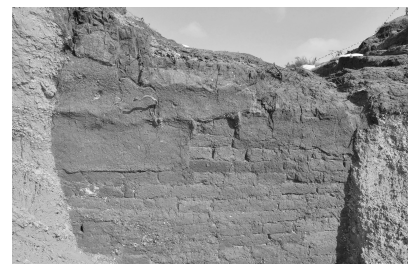
Fig. 23: Area B, the mud plaster, covering the upper courses of the fortification wall.
