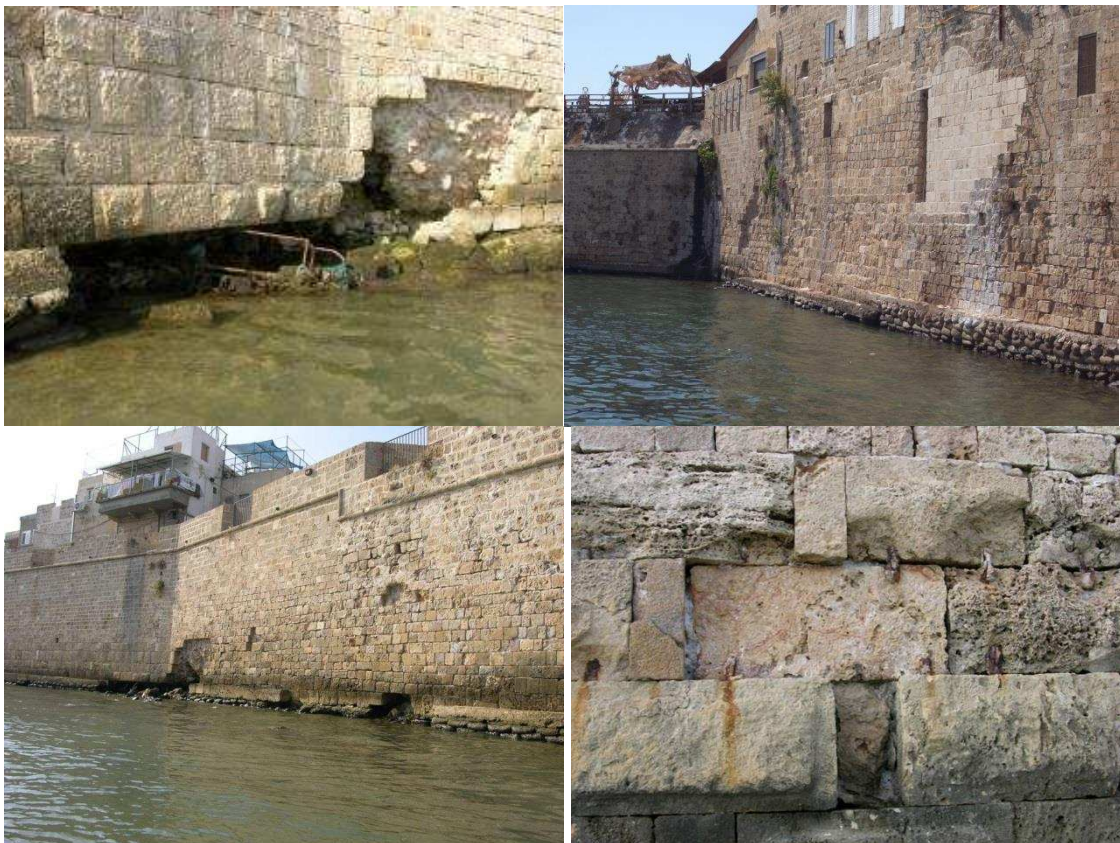
Fig. 1a, 1b, 1c,1d Part of the engineering failures of the sea wall
