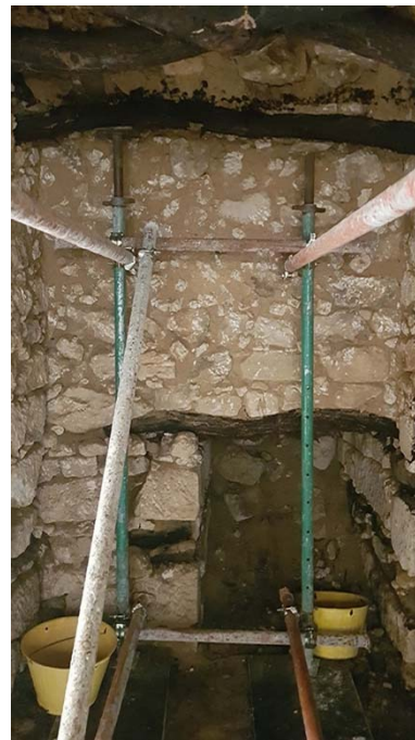
Fig. 10 - Consolidation works at the second storey of the citadel, June 2019 (Photo by A. Gratteri).
