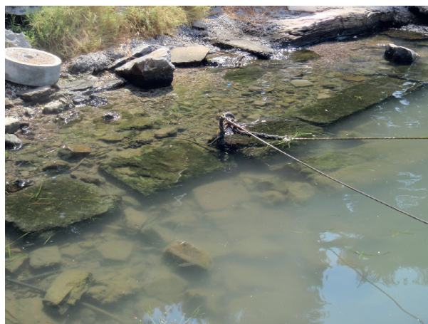
Figure 4.13: Frontal facade and walking level of the eastern quay-line, consisting of a single row of ashlar blocks and dressed stones (A. Ginalis).
