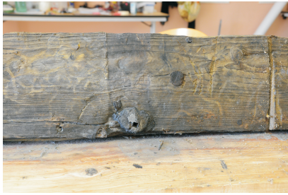
Fig. 11: Ceiling plank number 2: location of a treenail in the space between two frames. The nail is used to fasten the ceiling plank to a frame.
