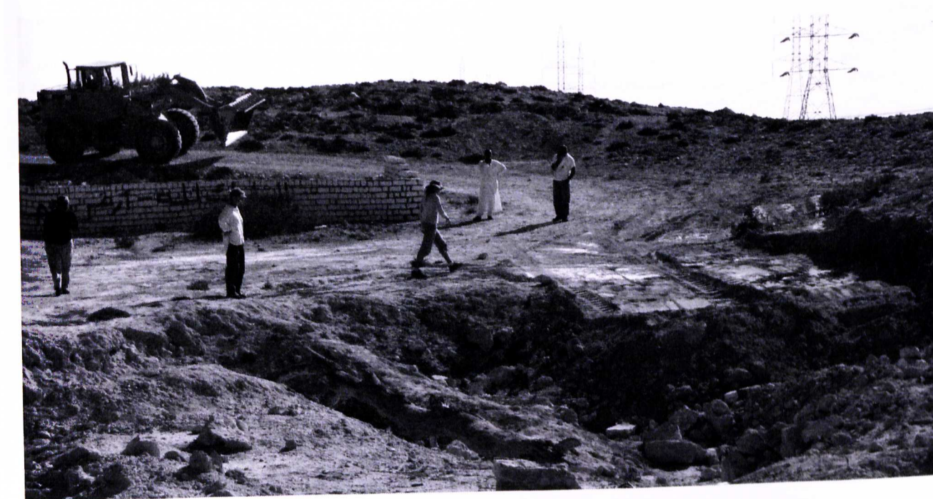
Fig. 12: Flattened Hellenistic tomb at Site 202 during bulldozer work in 2007 (Lake Mareotis Research Project).
