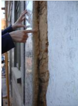
Fig. 3 Detachment of ceramic tiles and mortar
