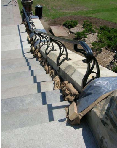
Fig. 11 Curing with wet burlap and plastic for a minimum of three days
