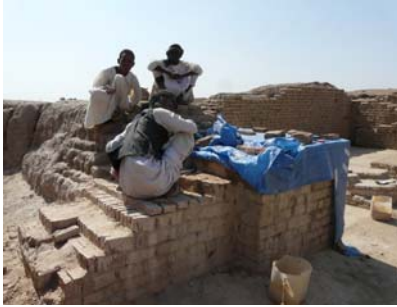
Fig. 7 Failed render to lower area of wall
