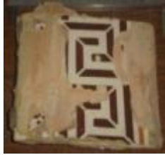
Fig. 5 Loss of glaze in a ceramic tile belonging to a façade
