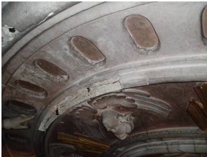
Fig. 5 Corrosion of metallic elements may require partial removing of the plaster
