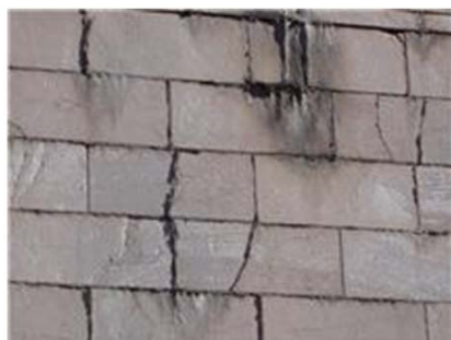
Fig. 16 Fissures due to constructive problems.
