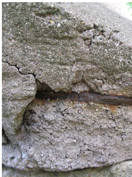
Fig. 2 Many busts have numerous cracks and cavities with visible corroded rods under a thin and porous mortar layer
