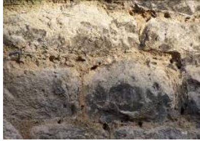
Fig. 9 Mud-mortared limestone exterior, Malton. To be limewashed rather than repointed with lime to avoid loss of earth mortar
