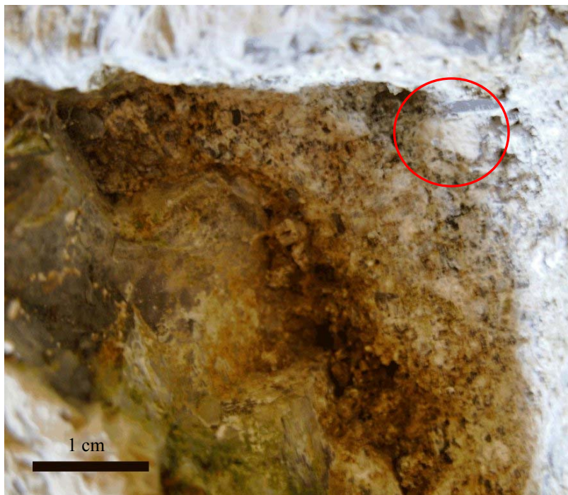
Fig. 1 Mortar joint with lump of lime (upper right corner, inside the red circle)
