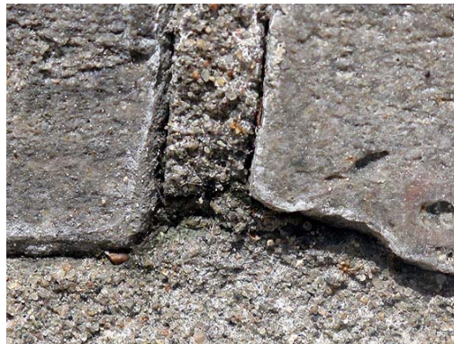
Fig. 9 Condition of joint mortar in Spring (Canada)
