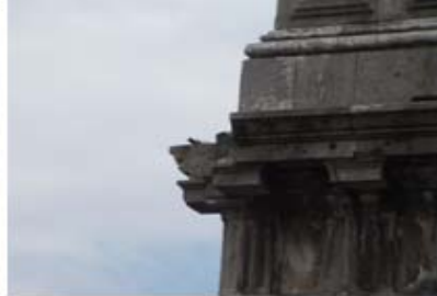
Fig. 8 Missing elements of decoration
