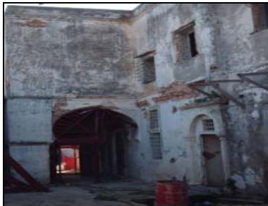
Fig. 6 Moisture in the external wall
