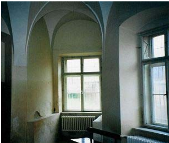
Fig. 2 The original condition of the wall in the interior of the library before renovation actions in 2001
