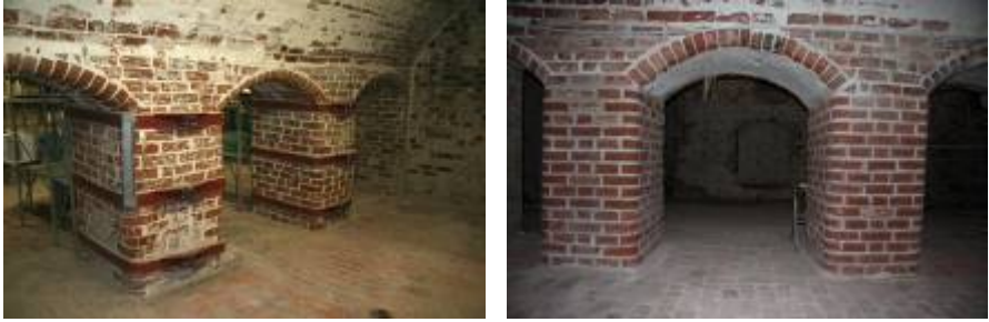
Fig. 10 Pillars in the basement of the city hall Lüneburg. Left: Situation before start of repair work. The masonry consists of brick and gypsum mortar. The pillars are safeguarded by steel profiles; Right; Pillars in final state, rebuilt using high fired gypsum mortar
