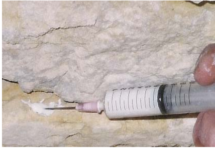
Fig. 5 St. Peter in Aachen-Orsbach, - residues of mortar were stabilised using injection masses
