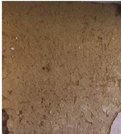
Fig. 5 York House interior, earth plaster, surface as produced by opening up of float before limestone dust and lime-rich finish coat applied over
