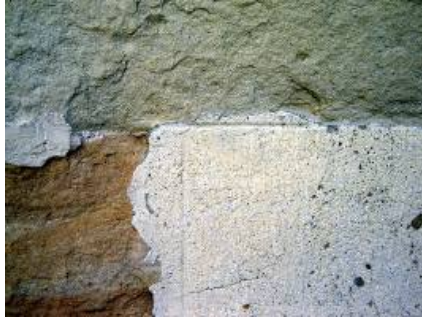
Fig. 4 Surface repair of a stone masonry. The repaired surface is durable but stone continues to decay. Aesthetically it is not functioning very well and it could accelerate decay of the adjacent stone.
