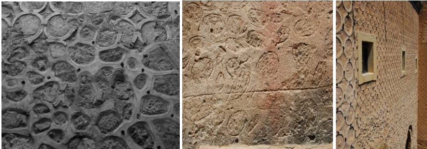
Fig. 11 The effects of the plaster work on joints in a non-plaster masonry walls. This could evolved towards sgraffito; Figs. 12 and 13 Sgraffito in Segovia, Spain
