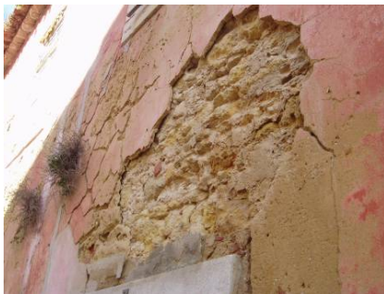
Fig. 7 Mechanical damage due to incompatible new render
