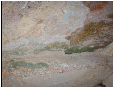
Fig. 5 Lichen on the external wall
