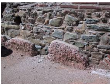
Fig. 6 Thick render in a wall during the Roman period (Olynthos 4 th century B.C.).
