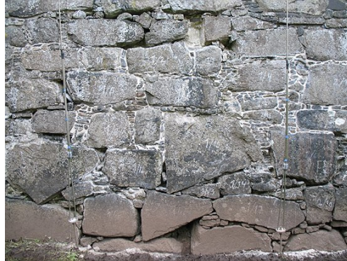
Fig. 2 The walls of the cathedral are made of irregular basalt boulders. The cavities in between are filled with smaller pieces of rock held in place by the mortar. Test area for restoration on the north side of the north wall
