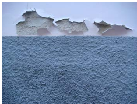
Fig. 3 The deterioration of cement plaster at Rui Barbosa's House
