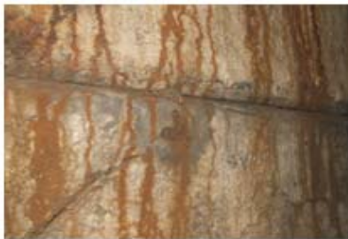
Fig. 7 Stains of oxide
