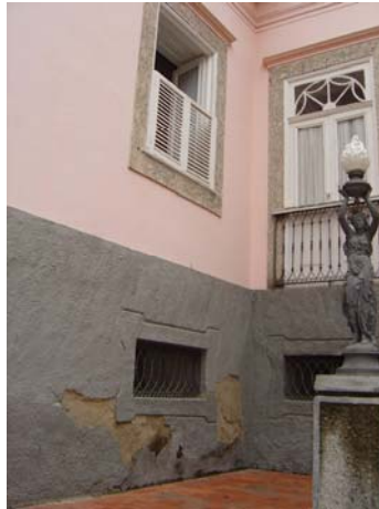
Fig. 2 The deterioration of cement plaster at Casa de Rui Barbosa Museum
