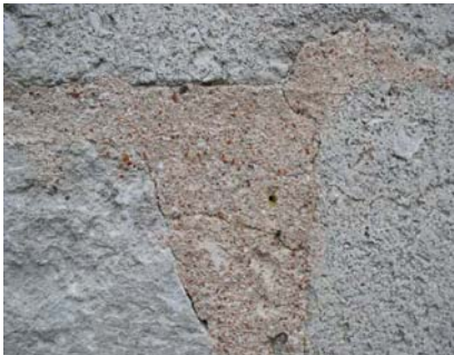
Fig. 5 Joint on Fardhem church containing crushed red bricks. Pink secondary mortar based on lime.
