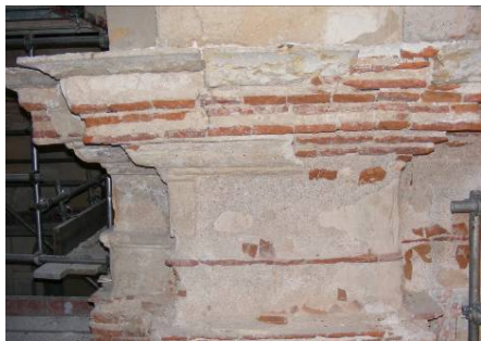
Fig. 10 Detachment of the mortars, showing the brick structure.
