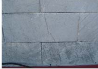
Fig. 4 Fissures in stone cladding
