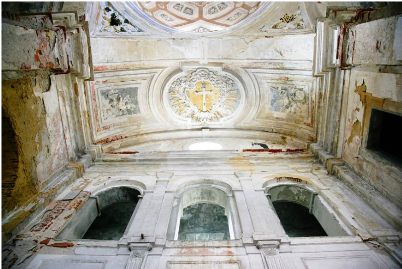
Fig. 9 Degradation observed on the decorative layers.
