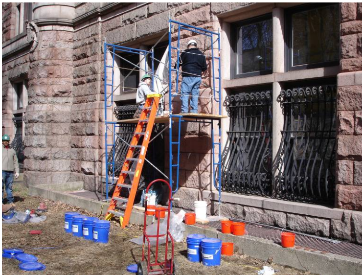
Fig. 6 Masons preferred the workability of natural cement mortars to portland-lime, when both types were installed in mock-up areas.
