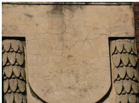
Fig. 1 Typical irregular network of fine shrinkage cracks characteristic of Roman cement stucco.
