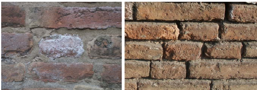
Fig. 6 Differential efflorescence in the bricks (left) and salt decay in correspondence to the mortars (St. Lazarus church in Modena, Italy, XII-XVII cent.)
