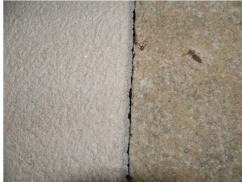
Fig. 21 Repair mortar (left) versus original stone (right).
