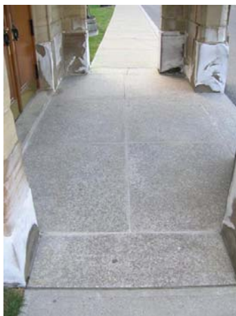
Fig. 6 Floor paving subject to severe exposure. Note salt saturation from de-icing salts at the bottom of the columns (side entrance Parliament buildings, Ottawa, Canada)
