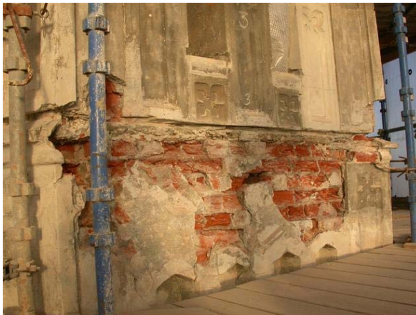
Fig. 4 The damage on the bricks underneath the open walkway in the tower
