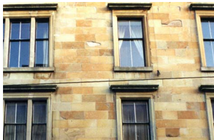
Fig. 1 Advanced deterioration of the 19th century sandstone ashlar masonry façade.
