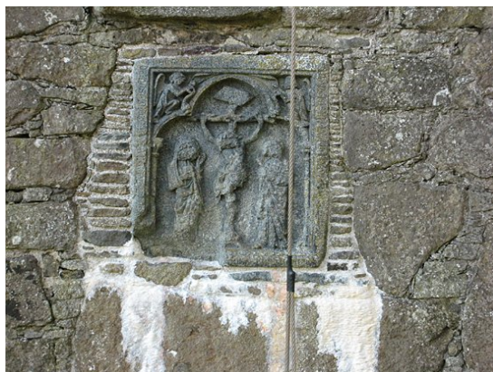
Fig. 5 The lime deposit below the relief on the east wall has leached from the lime mortar used for the joints.
