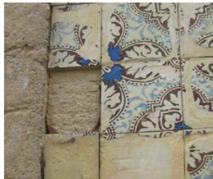
Fig. 4 Lack of ceramic tiles
