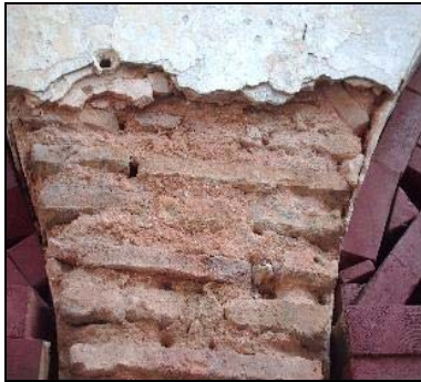
Fig. 4 Detachment of cement mortar
