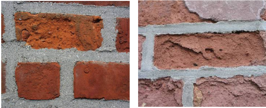
Fig. 4 Salt damage as a result of the application of a water repellent
