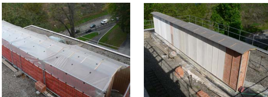
Fig. 2 External masonry brick wall showing the protective covering (left side) and the different coatings (right side)
