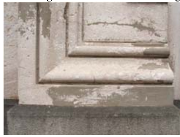
Fig. 6 Previous repair mortars
