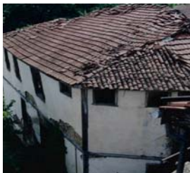
Fig. 1 The storehouse before collapsing
