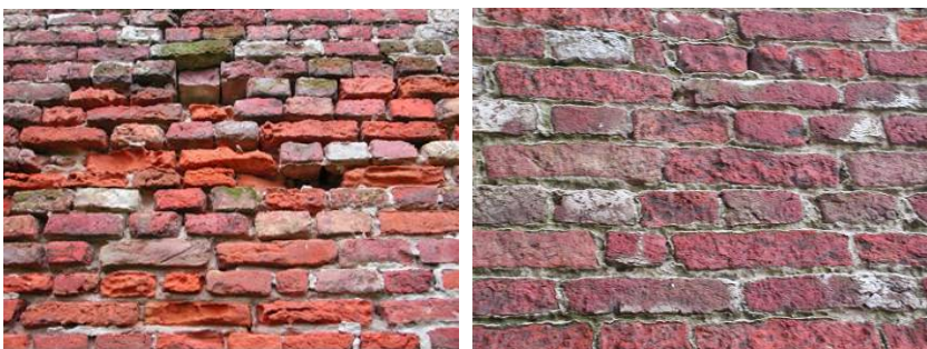
Fig. 2 Examples of the damaging effects of sea salts on respectively masonry and in lime mortar joints (pitting in the pointing mortar).
