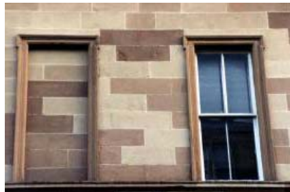
Fig. 2 Example of mortar application as a surface repair of deteriorated stone units.
