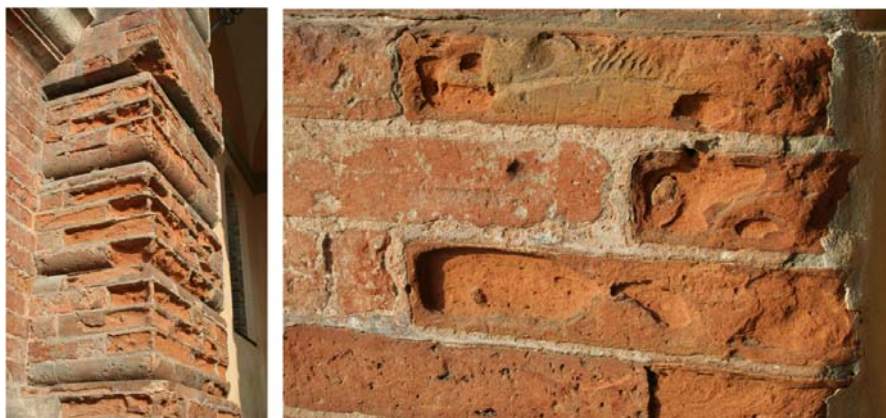
Fig. 2 Details of the materials' decay in the portal
