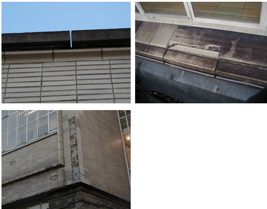
Fig. 2 Different risks for water infiltration: missing joints between covering stones (top left), defects in window sills (top right), missing tiles (bottom left).
