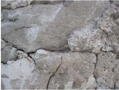
Fig. 3 Two types of old mortar on the west façade of Othem church. They are both white and lime rich. One with fine graded sand and the other with larger rounded sand particles.
