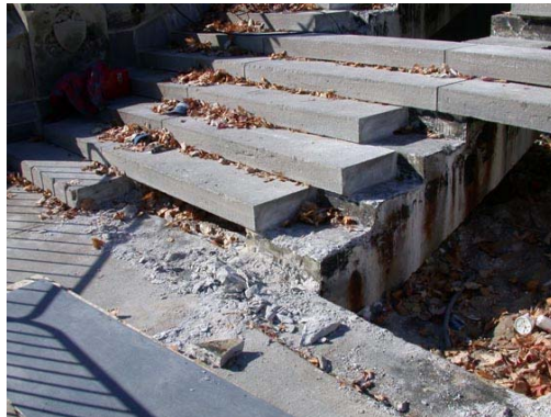
Fig. 10 Salt damage on mortar, stones and concrete base of stairs. Partial dismantling (Canada)
