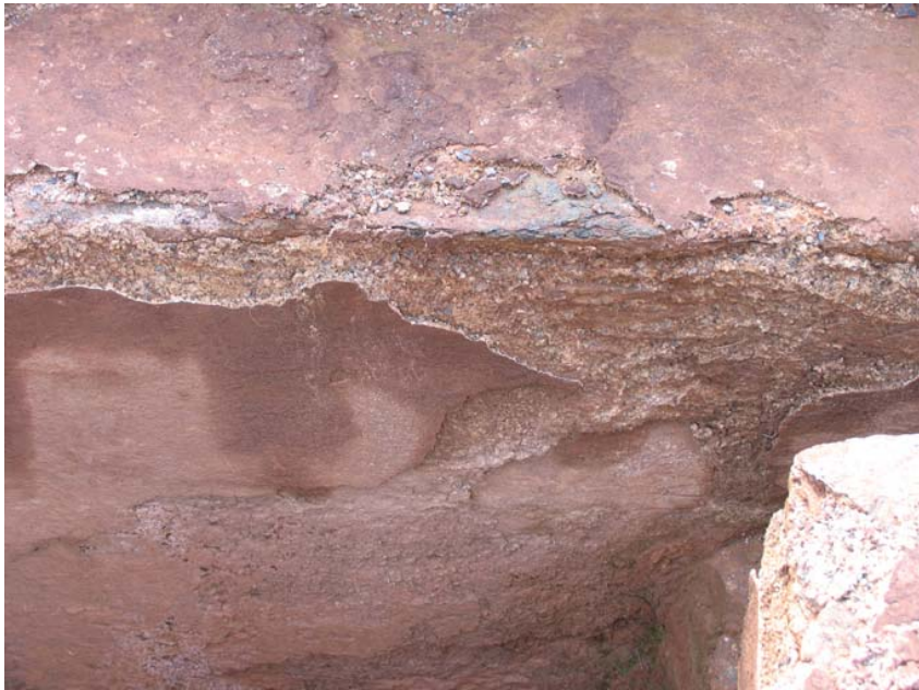
Fig. 1 Plaster at the edges of the floors is most prone to deterioration caused by water ingress.
