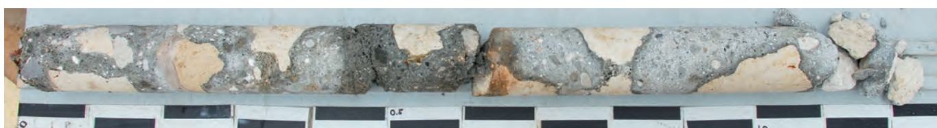
Fig. A3.74: ALE.2007.03, detail, 0 to -1.20 m. Oolitic limestone and occasional ceramic caementa, and compact mortar with greenish-gray pumiceous ash pozzolan and relatively few relict lime clasts. Scale bar is 10 cm.
