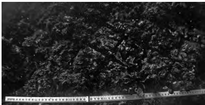
Fig. 8.2. Opus reticulatum facing on the sides of a concrete pila at Secca Fumosa near Baiae.
