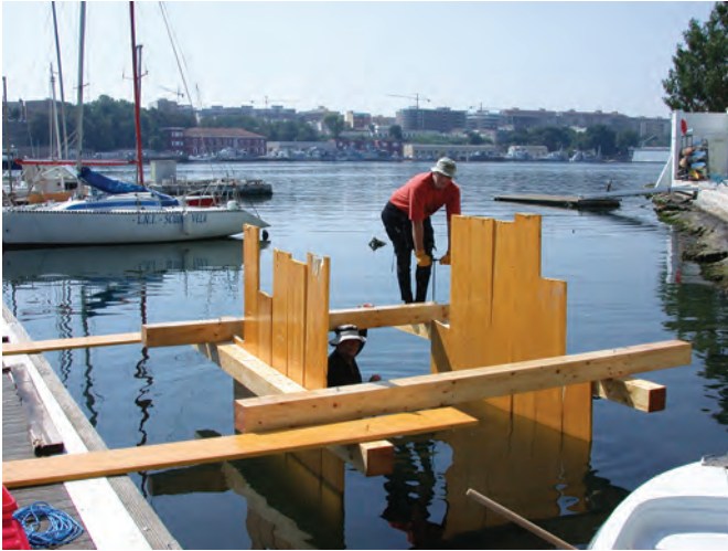
Fig. 5.6. First two plank walls in position; bolt hole being drilled in horizontal collar beam joint.
