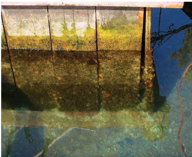
Fig. 5.22. Condition of the formwork planks at low tide, November 2005.
