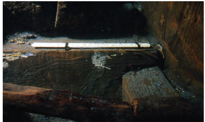
Fig. 8.27. Detail of the fixing bracket securing the lower rail to a stipes on the formwork on the side of a concrete quay to the South of Punta Pennata at Misenum (Benini and Lanteri 2010: fig. 14; used with permission).
