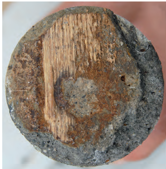
Fig. A3.73: ALE.2007.02, detail of base of core, -1.03 m. Wood from formwork.
