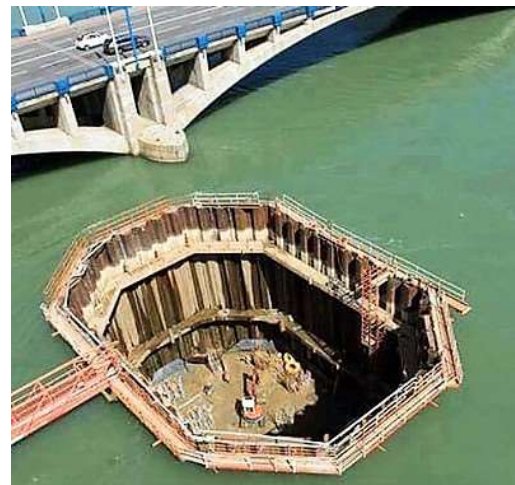
Fig. 36. Cofferdam on the Godavari river for the Polavarán irrigation project (Hans India 2017)
