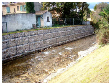
Fig. 46. River bank protection with gabions made of steel wire and filled with small rock ( https://www.lacompagniedesforestiers.com )
